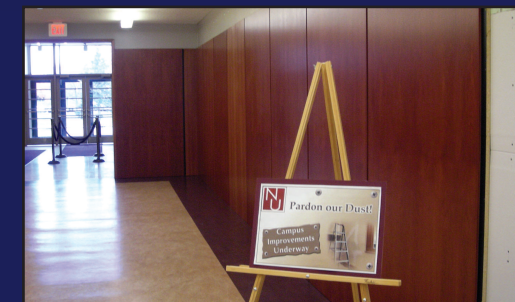
Renovations to Janse Hall's main floor in Lombard continue with the removal of lockers and addition of paneling.
