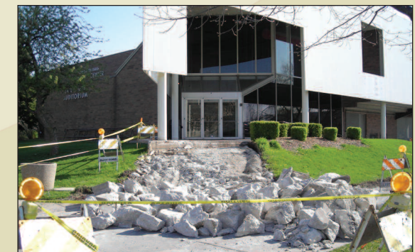
Freshly laid concrete can be found in several locations around campus including the steps outside the Student Center.
